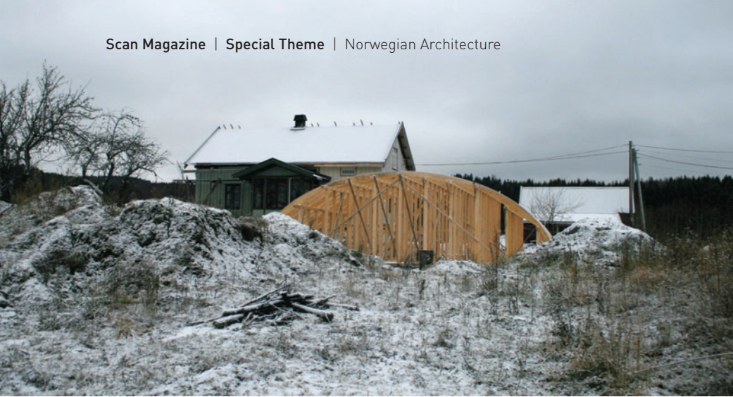
Senstad construction. The practice is currently building a new farmhouse in Senstad, about an hour outside Oslo. The vision is to integrate the new house into the farmland without disturbing existing historic farm buildings or the scenery. The new house is being built into the ground, with a grass roof designed as a slight hilltop in the garden. This building has been tailored to the family's as well as the farm's basic needs.
